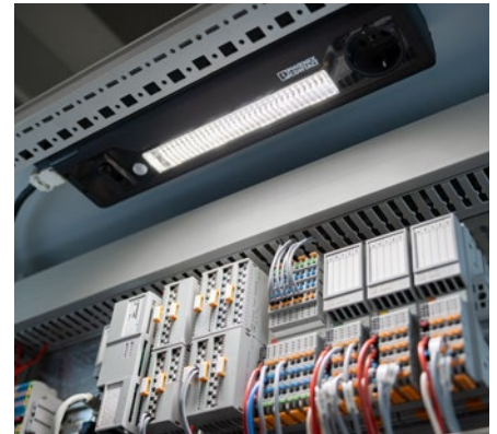
AC light mounted in the control cabinet.
