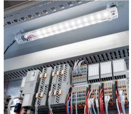
Standard light mounted in the control cabinet
