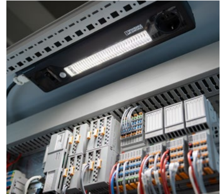
AC light mounted in the control cabinet
