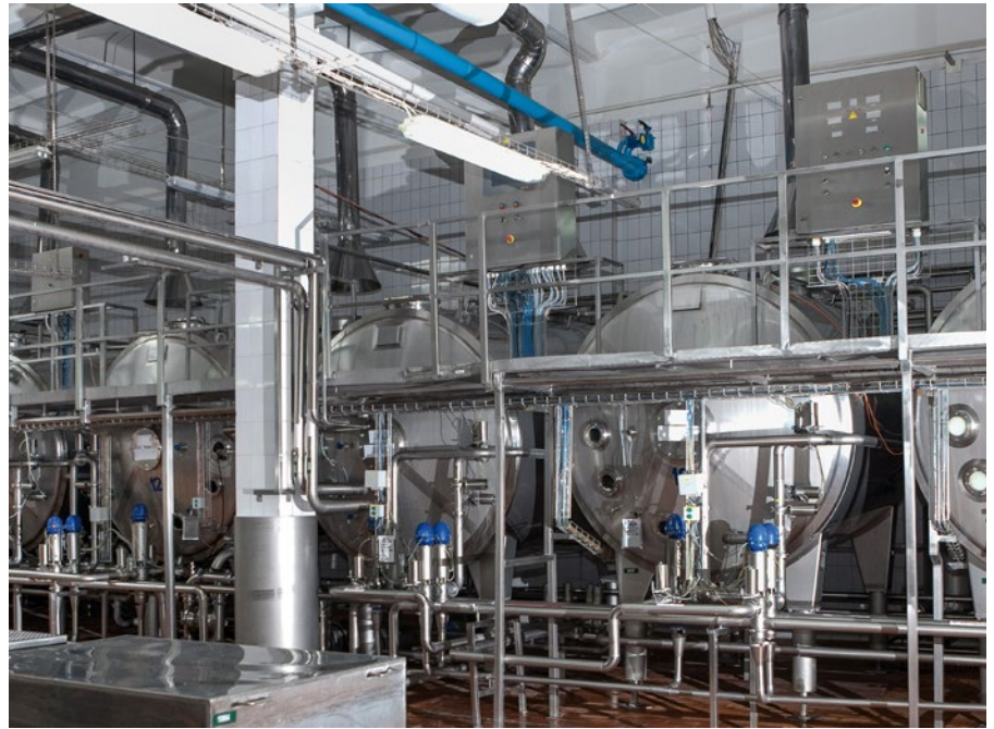
Processing plant in the pharmaceutical industry with various loads
